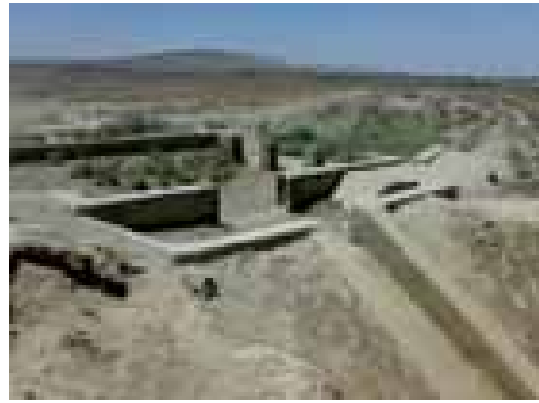
Figure 4.6: Division box at branch canal 5
