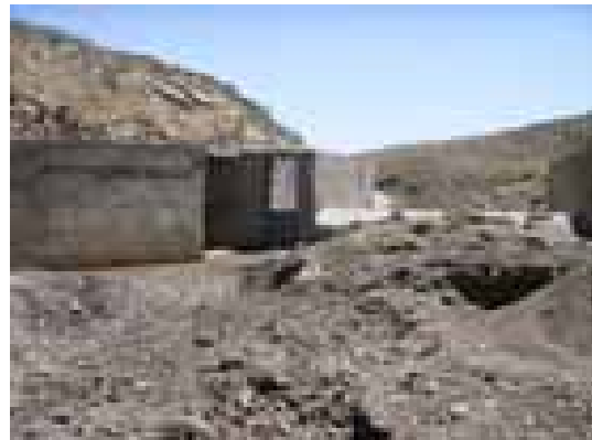
Figure 4.8: Sedimentation at the headworks
